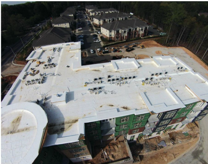
QUANTITY AND QUALITY: Space conditioning at the new facility is achieved with 68 condensing units on the roof and 145 evaporators throughout.
