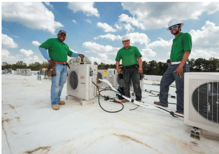
A TEAM EFFORT: employees at Raleigh, North Carolina-based Eco Green Air install one of many rooftop condensing units at the Chatham Pointe development in Cary, North Carolina.
