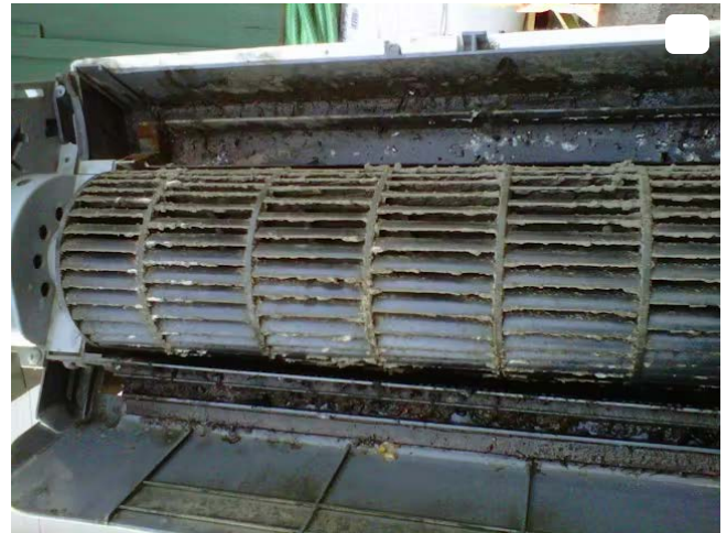
Dust more readily adheres to fan wheels because they're on the cool side of the system.
