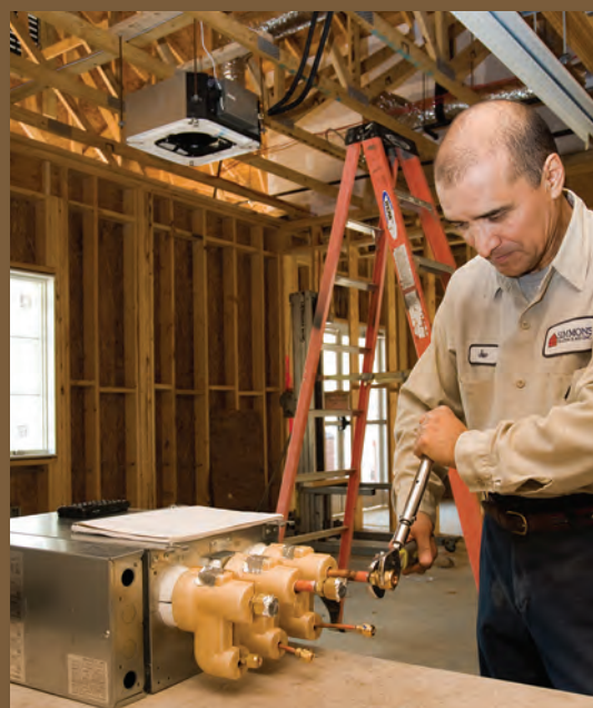
A technician prepares refrigerant lines for a ceiling cassette in the addition at Cornerstone Church, California, MD.
