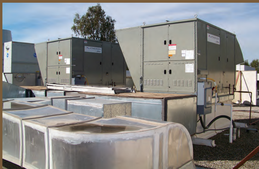
Modine's Atherion commercial packaged-ventilation system, a 100% dedicated outside-air system with an integrated energy-recovery ventilation (ERV) module, was installed at Rite Engineering, Franksville, WI, to improve temperature and air quality for the machine shop.
