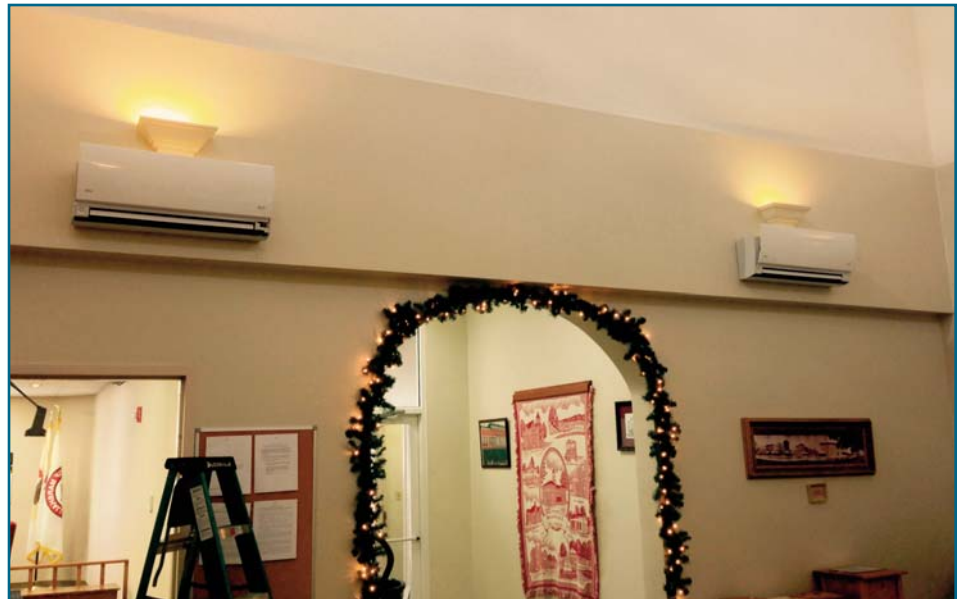
Below: Two 15,000 BTU/h RLS2-Series wall mounts were installed in the main area of the City Hall. These system are extremely energy efficient due to their high SEER ratings and ductless technology.
