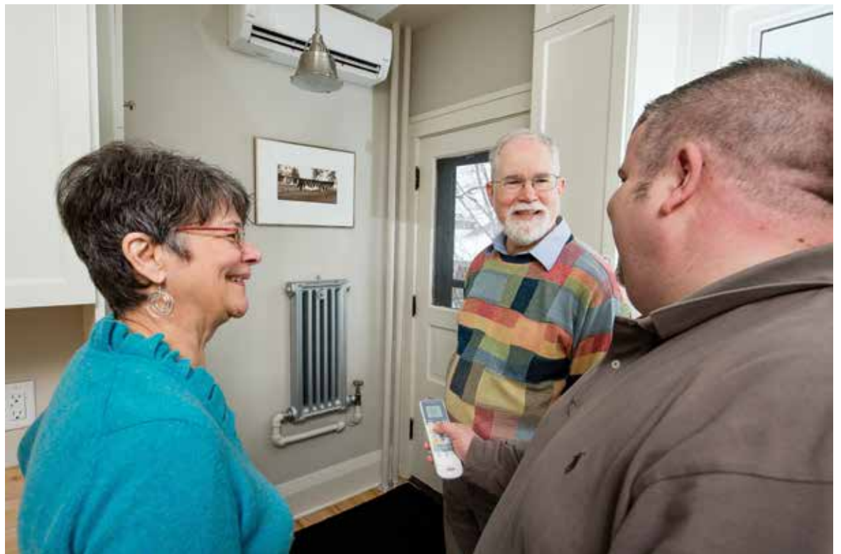
Nick Steckahn, president, Aabott Ferraro (right), introduces Nancy and Bill Rouner to one of the wireless remotes on their newly installed heating and cooling system.
