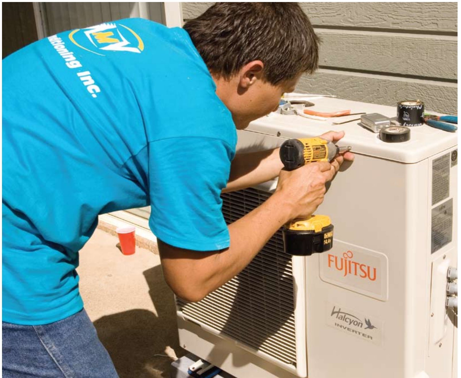
Billy Souza, installation supervisor, at AMV Air Conditioning, Inc., sets the outside unit of the Fujitsu ductless system.
